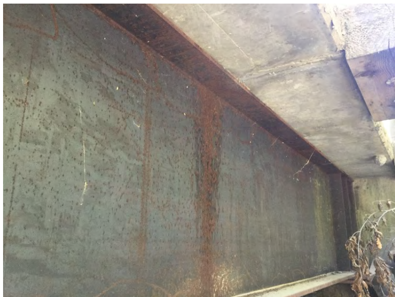
Evidence that water is getting through deck joint
