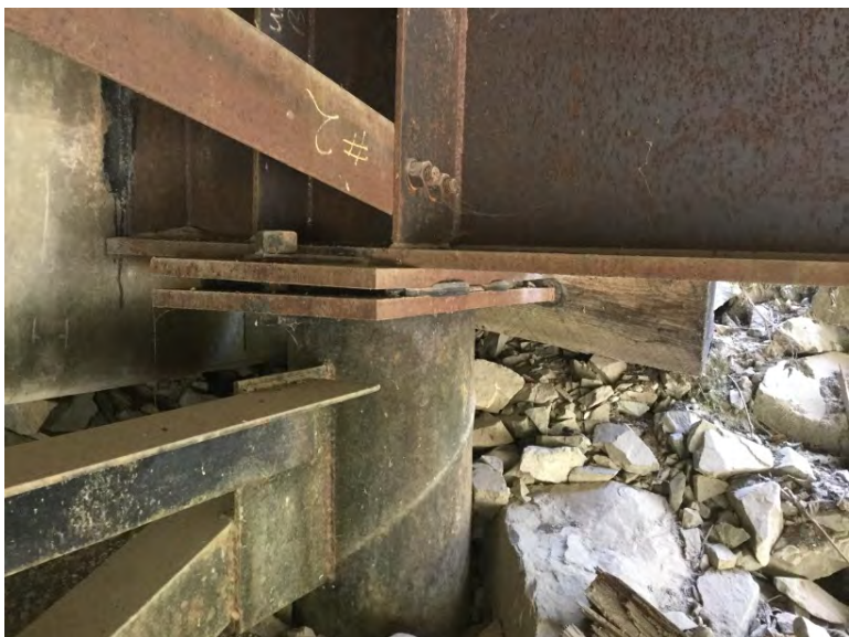
Slight bulging of bearing pads at left bank
