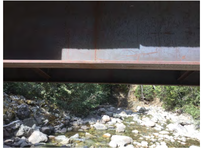
Slight deformation on bottom flange - at weld location
